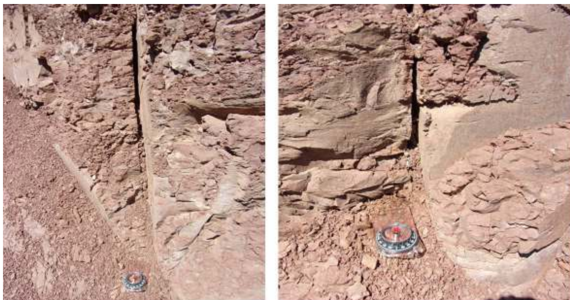
Fig. 14. Open joint trending N-S observed in the bank of the road at Les Détroits Pass, as described by Ballantyne (1996). We must be cautious for possible displacement of the blocs when making the road or due to movement on the slope. Here the trend of the joints is parallel to the slope and orthogonal to the road, and blocks extends on both sides over tens of meters.
